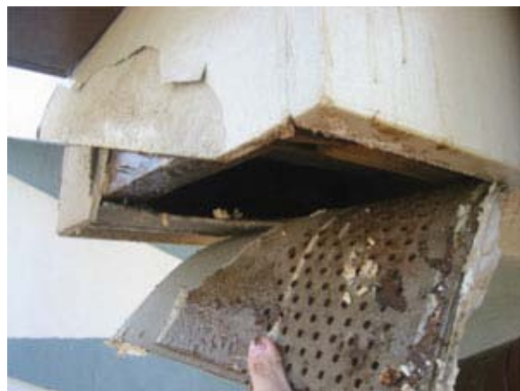
Building envelope moisture entry [Aldous 2008]
