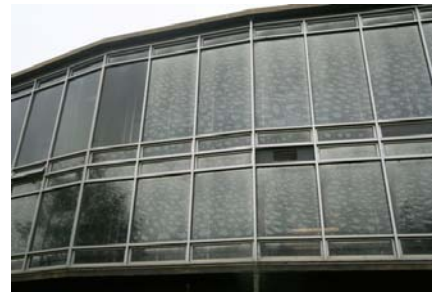
Failed window film treatment.
